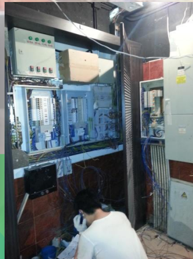
空制箱及設備測試 Equipment Testing
